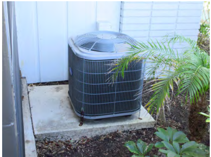
GENERAL VIEW OF HVAC EQUIPMENT
