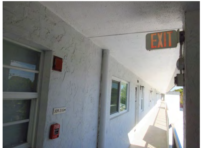
VIEW OF LIFE SAFETY EQUIPMENT
