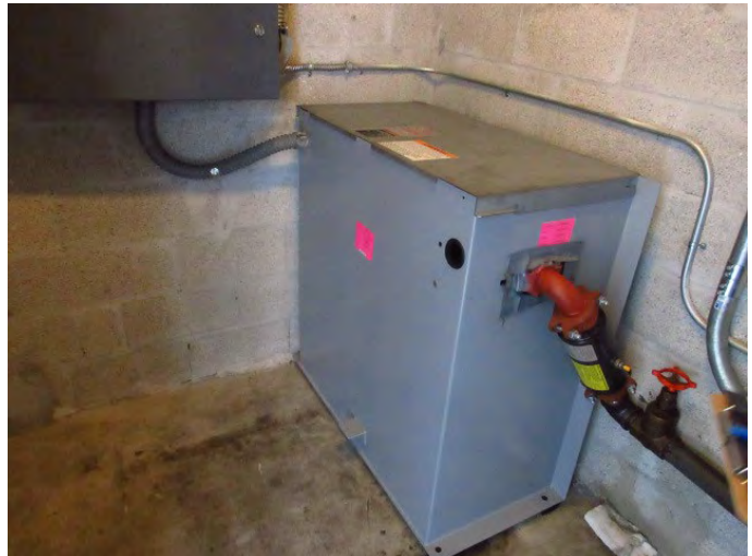
VIEW OF ELEVATOR EQUIPMENT
