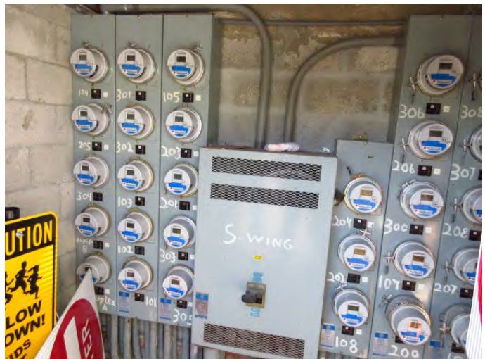
VIEW OF ELECTRICAL EQUIPMENT
