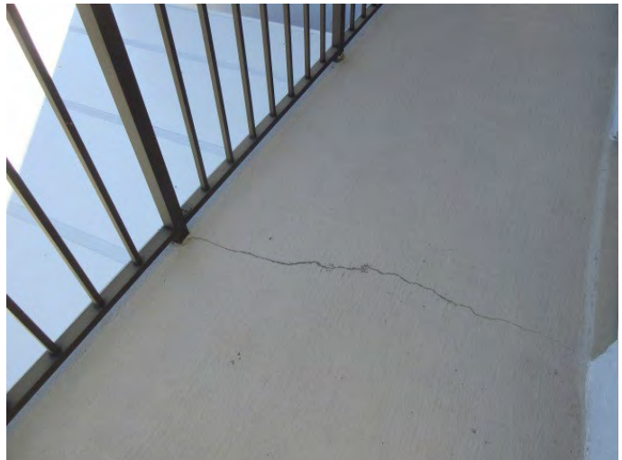
VIEW OF CRACK AT ELEVATED WALKWAY
