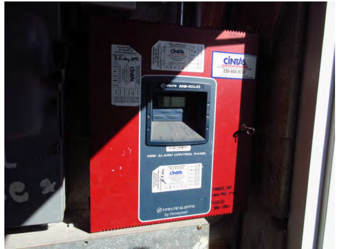
VIEW OF CENTRAL ALARM PANEL
