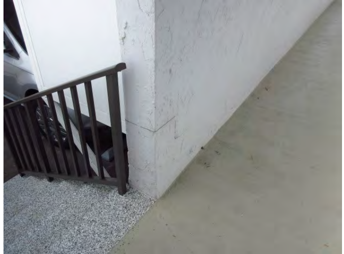
VIEW OF CMU STEP-CRACKING
