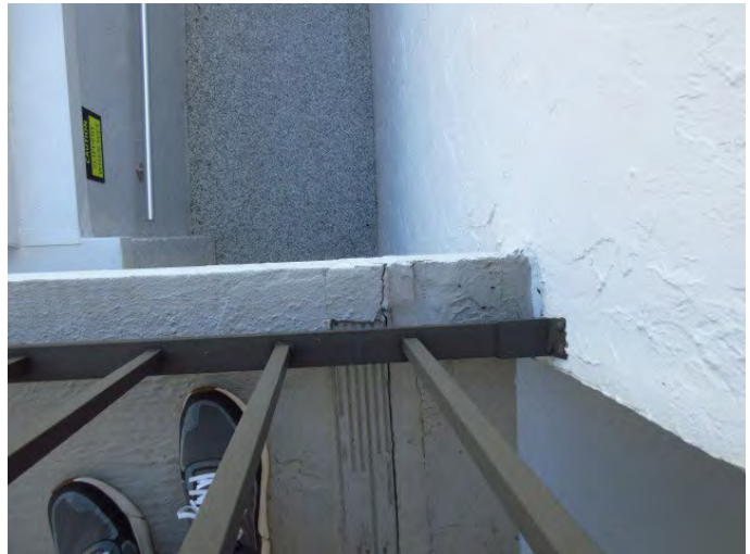
VIEW OF FAILING EXPANSION JOINT
