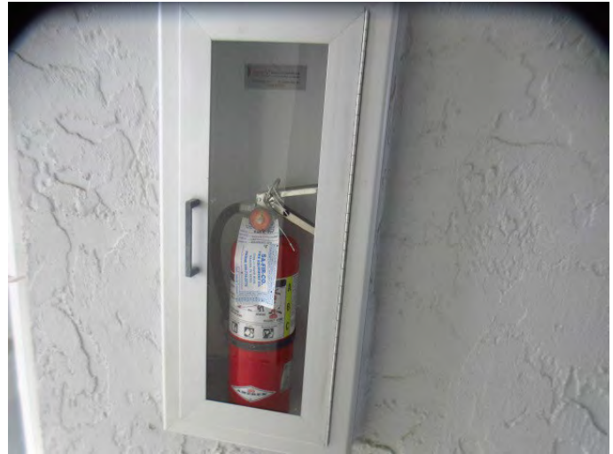
VIEW OF FIRE EXTINGUISHER
